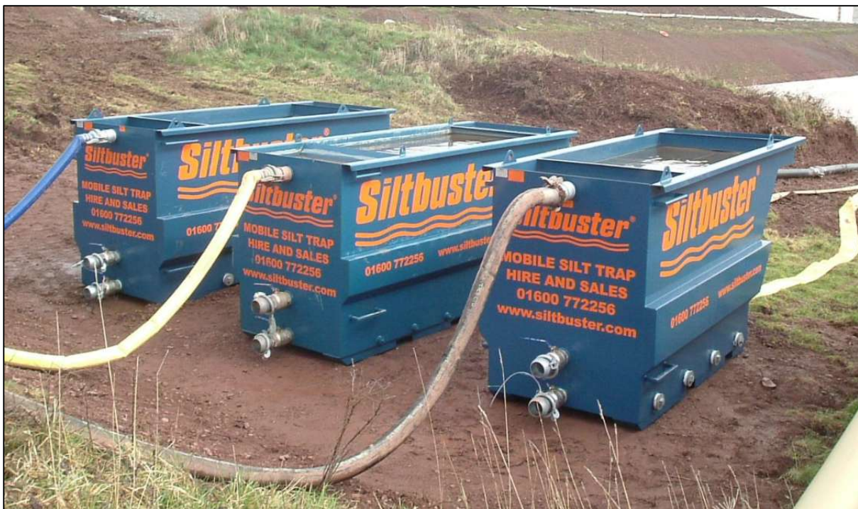
Figure 5-4: Temporary site settlement tanks (Source: Siltbuster)
